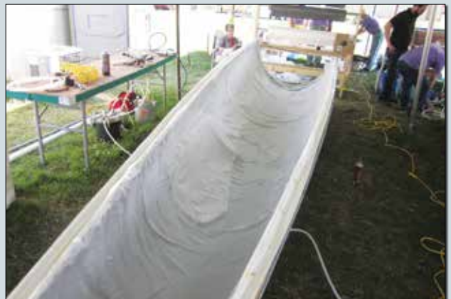
...the peel ply can be added, trimmed, and tacked down at the edges, just outboard of the MTI hose.
