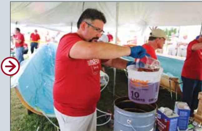
Jeff Starcher, from resin supplier Scott Bader Company Ltd., serves as mixmaster. This is Crestapol 1250LV, a tough, low-viscosity urethane acrylate resin designed for carbon fiber infusion. It is hardened with an MEKP catalyst, Triginox 239. Gel time at 77°F is 37 minutes, which tells a lot about how quickly the laminate will be infused.
